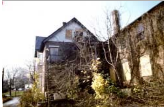
Boarding up without adequate ventilation and maintenance has accelerated deterioration of this property. Photo: NPS files.
