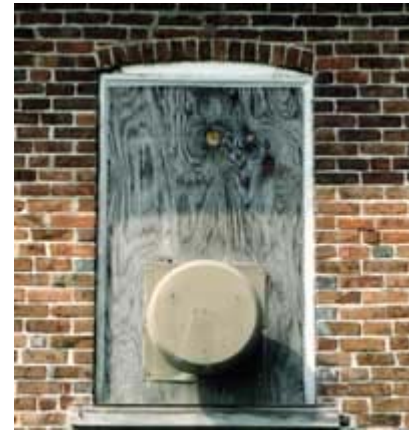
This exhaust fan has tamper-proof housing. Photo: Michael Mills, Ford Farewell Mills Gatsch, Architects.
