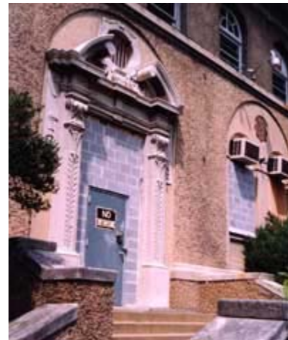
The first floor openings of this historic building have been filled with cinder blocks and the doors, window sash, and frames removed for safe keeping. The security metal door features heavy duty locks. Photo: NPS files.
